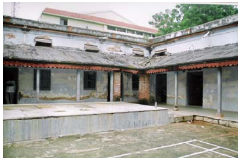
Dilapidated Government High School Building, Hanamkonda (Warangal District) certified to be not fit by the EE, R&B
